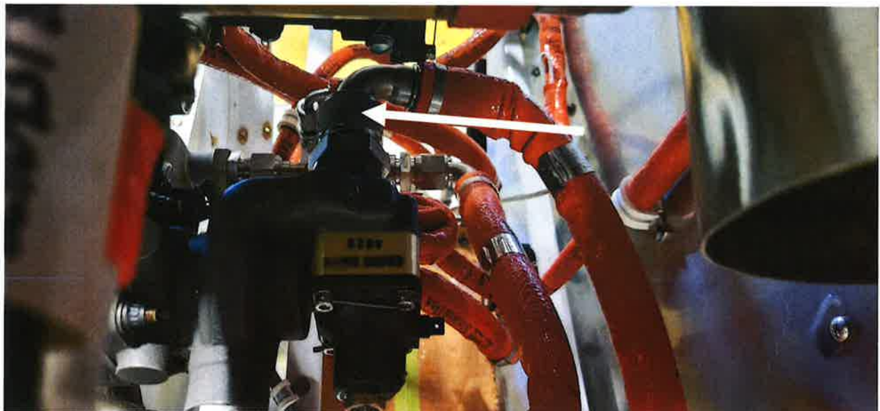
Figure 8.3.1.2 – Connection at Fuel Pump
